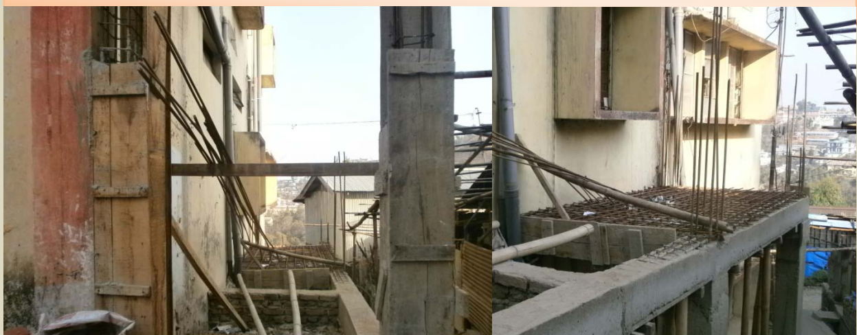
Construction of Ramp for differently abled persons in progress in the Directorate
