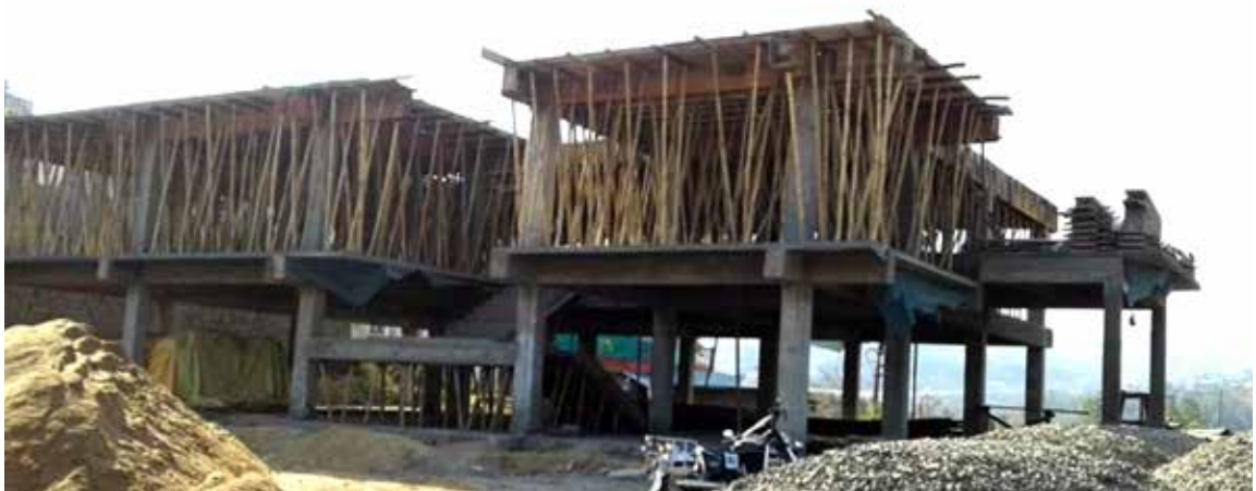
Construction of New Directorate Office building near the Nagaland Civil Secretariat, Kohima
