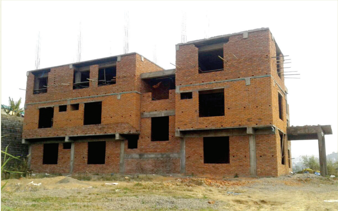
Constructions of New Directorate office Building near the Nagaland Civil Secretariat, Kohima
