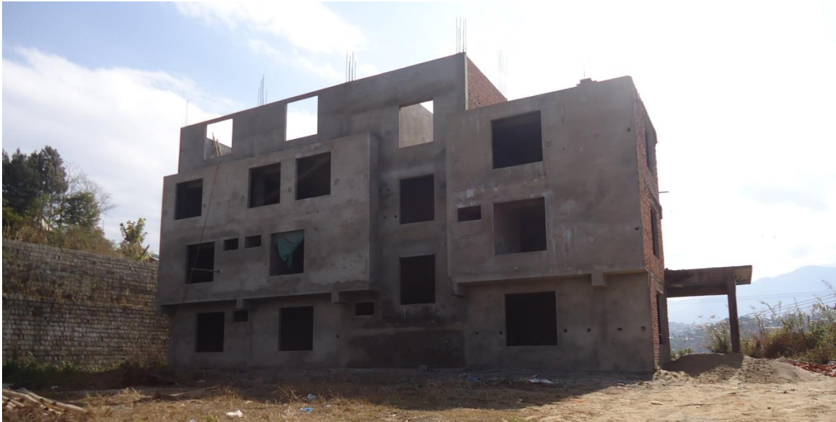
Constructions of New Directorate office Building near the Nagaland Civil Secretariat, Kohima.
